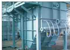
Dissolved Air Floatation Units
