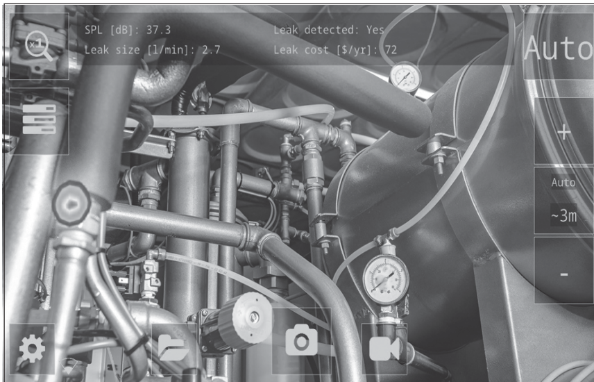
Industrial compressed air leak, as seen by the FLIR Si2-LD
