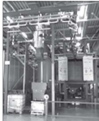
RHBD 13/18 Dust Collector System
